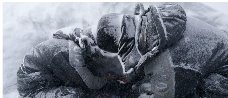
The emergency repair staff of the Chengde New Energy Business Unit of Datang Power checks the cable joints with bare hands in snow to guarantee electricity supply for every household.
