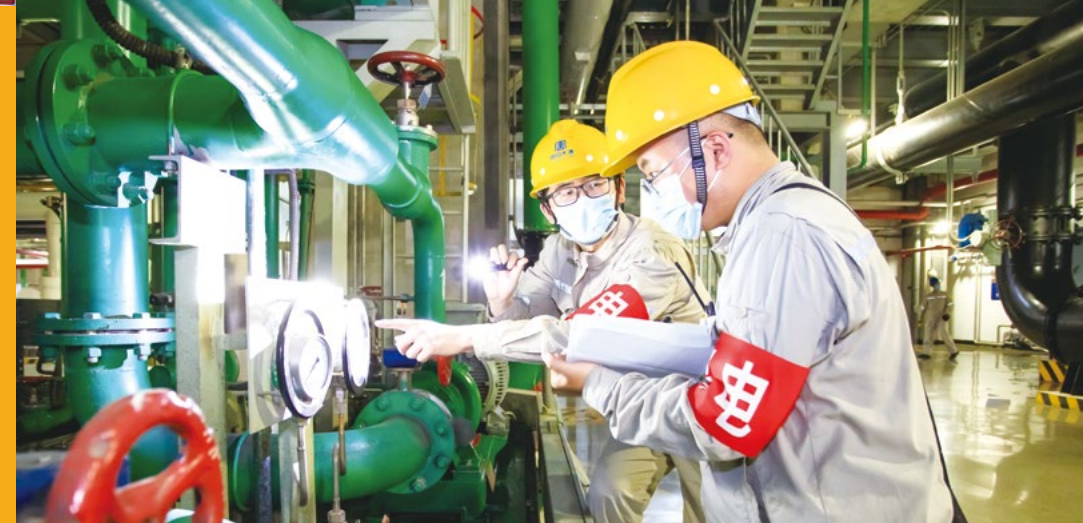
Inner Mongolia Datang International Tuoketuo Power Generation Co., Ltd. strengthens equipment inspection.
