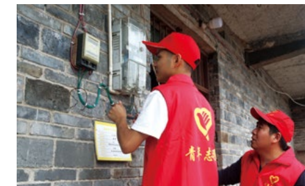
Village-based officials from Datang Chongqing Power Generation Co., Ltd. help a left-behind senior resident replace an old cable.
