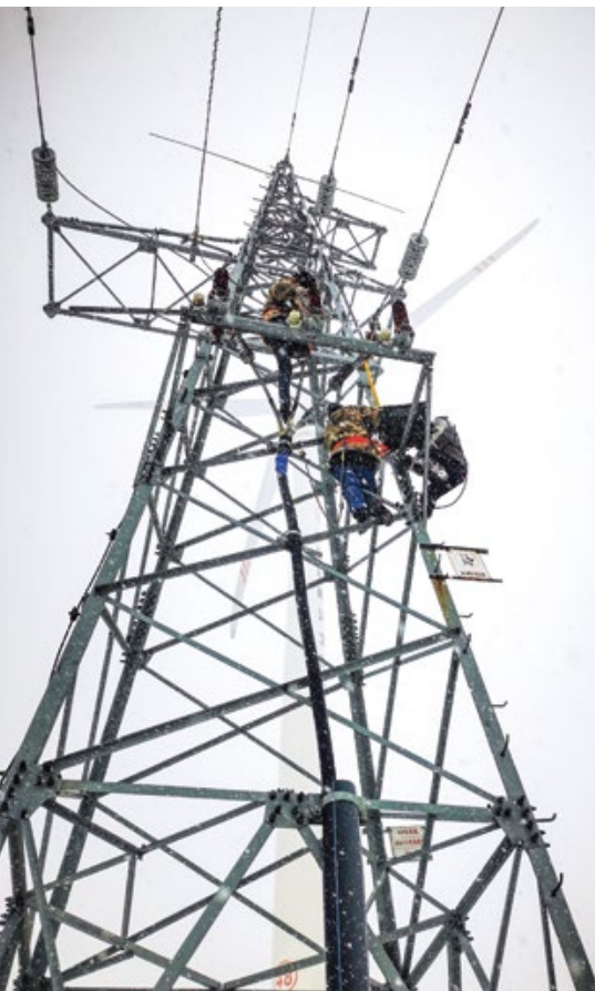
▲ Emergency repair staff from Chengde New Energy Business Division of CDT climb the tower on a windy and snowy day for an emergency repair mission.
