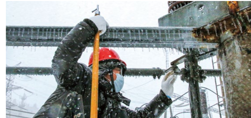
▲ Datang Jilin Power Generation Co., Ltd. makes every effort to cope with the extreme weather involving rain, snow, and freezing damage to ensure safe and stable heat and power supply in winter.
