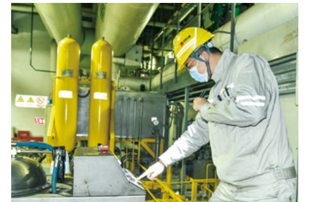
▲ A maintenance staff from CDT's Zhejiang Branch carefully inspects the equipment.
