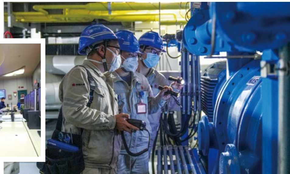
▲ Guangdong Datang International Zhaoqing Thermal Power Co., Ltd. makes every effort to ensure power supply for industrial parks.
