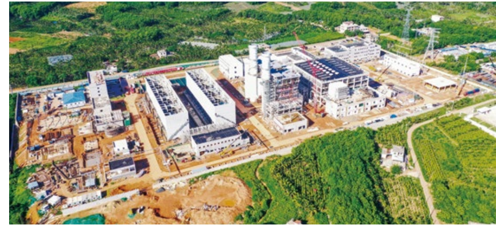
▲ Promoting the construction of the Wanning natural gas power generation project of Datang Hainan Energy Development Co., Ltd.
