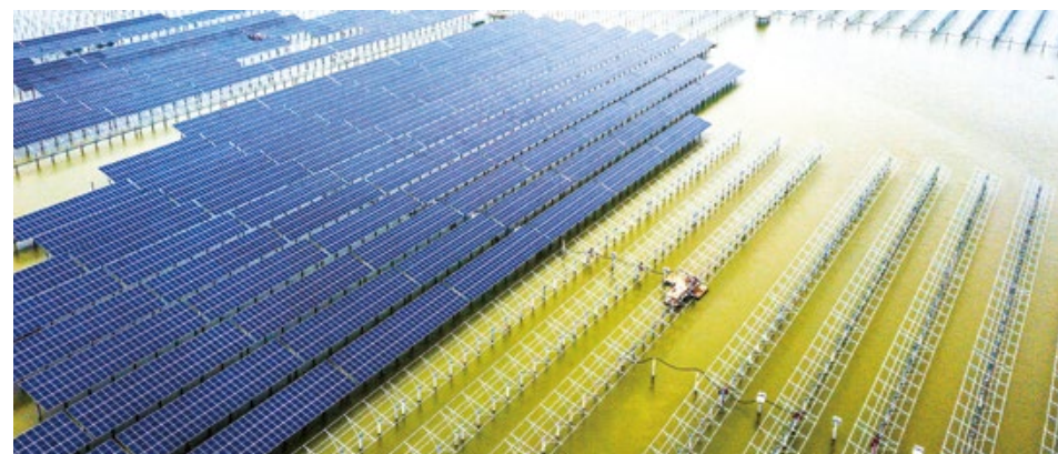
▲ Gaoan photovoltaic project of Jiangxi Datang International Renewable Power Co., Ltd.
